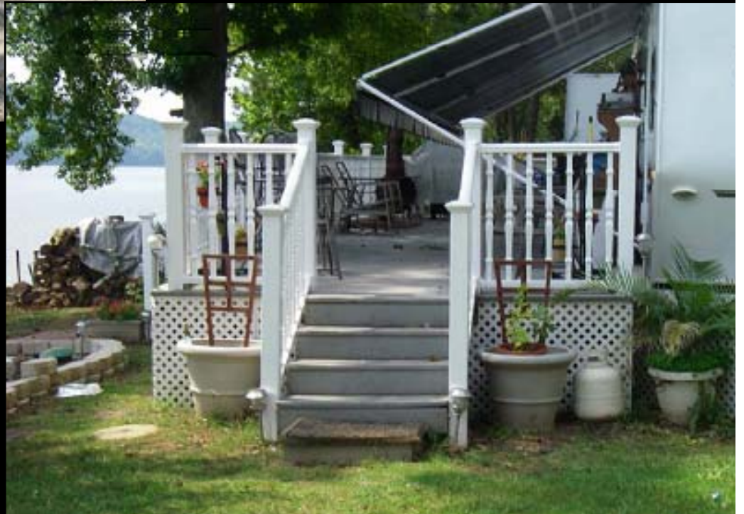
Long-term Permanent Use of Campsites and Safety Violations
